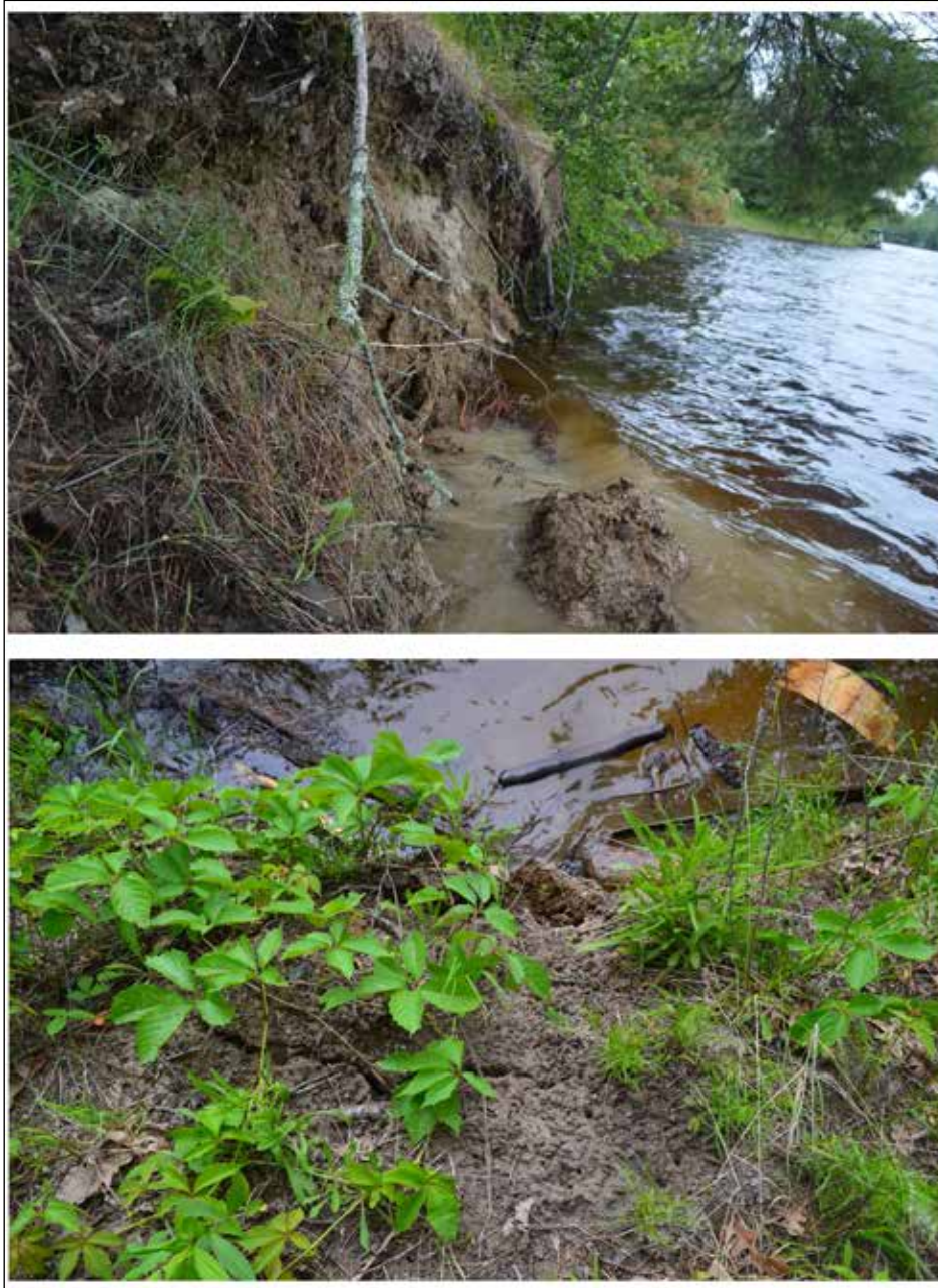
Figure 15. Erosion at sites 21SL51 (top) and 21SL53 (bottom), June 2014.
