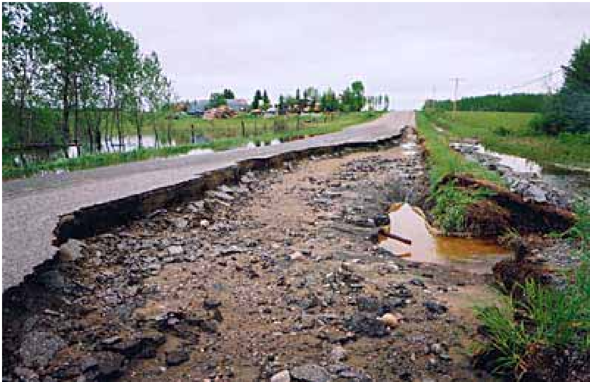
Road Washout West of Fort Frances, Ontario Photo Courtesy of Fort Frances Times
