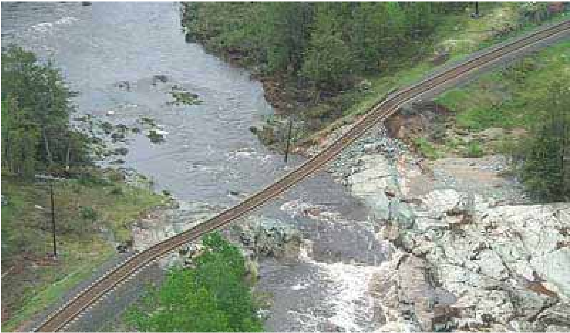
Railway Washout East of Fort Frances, Ontario Photo Courtesy of Canadian National Railway Company
