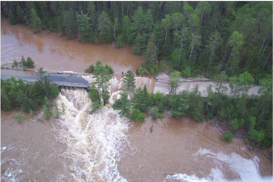
Bridge on Turtle River in Ontario Photo Courtesy of Ontario Ministry of Natural Resources
