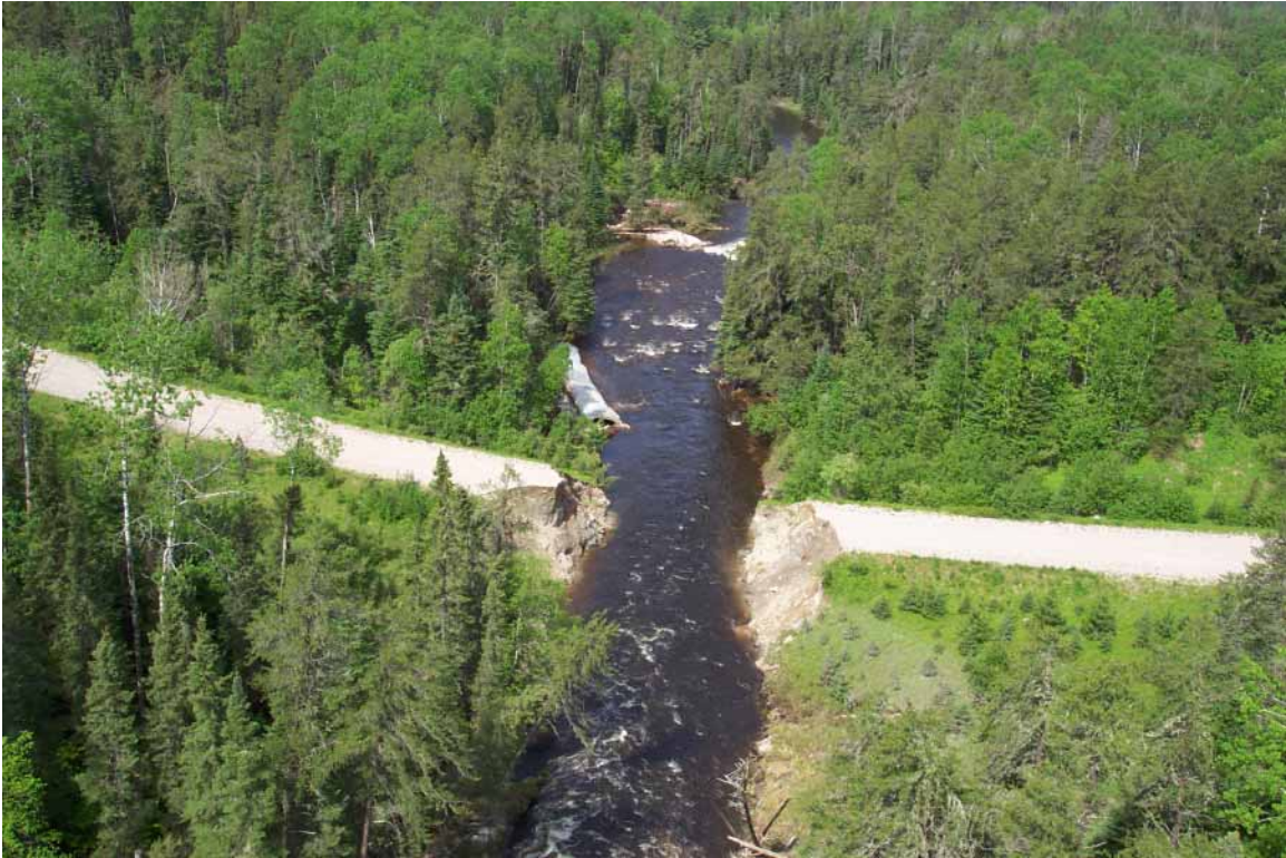
Road Washout East of Fort Frances, Ontario Photo Courtesy of Ontario Ministry of Natural Resources
