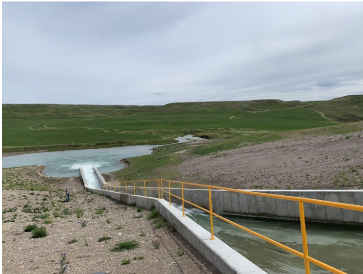
U.S. St. Mary Canal hydraulic drop structure #5
