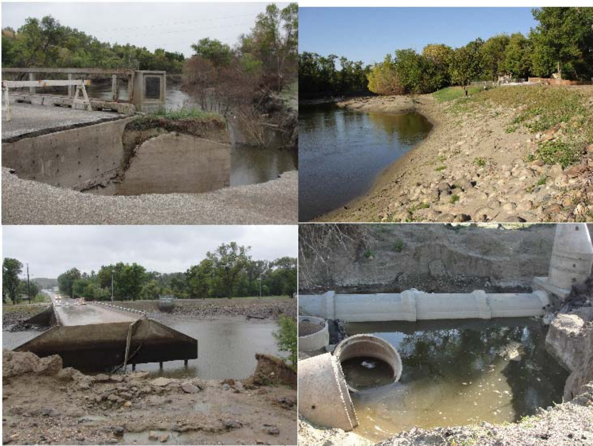
Above - left to right: damage to public infrastructure
