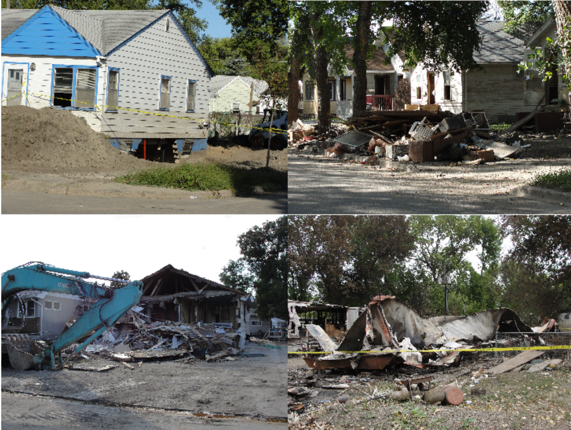
Above - left to right: basement damage; contents of home awaiting debris removal; home being demolished; inundated trailer home after gas fire.
