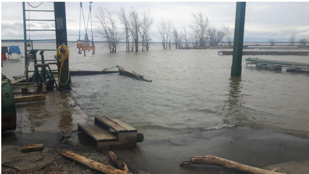
Image 4: Flooded and damaged service dock (Photo Credit: David Speak, Beaconsfield Yacht Club)
