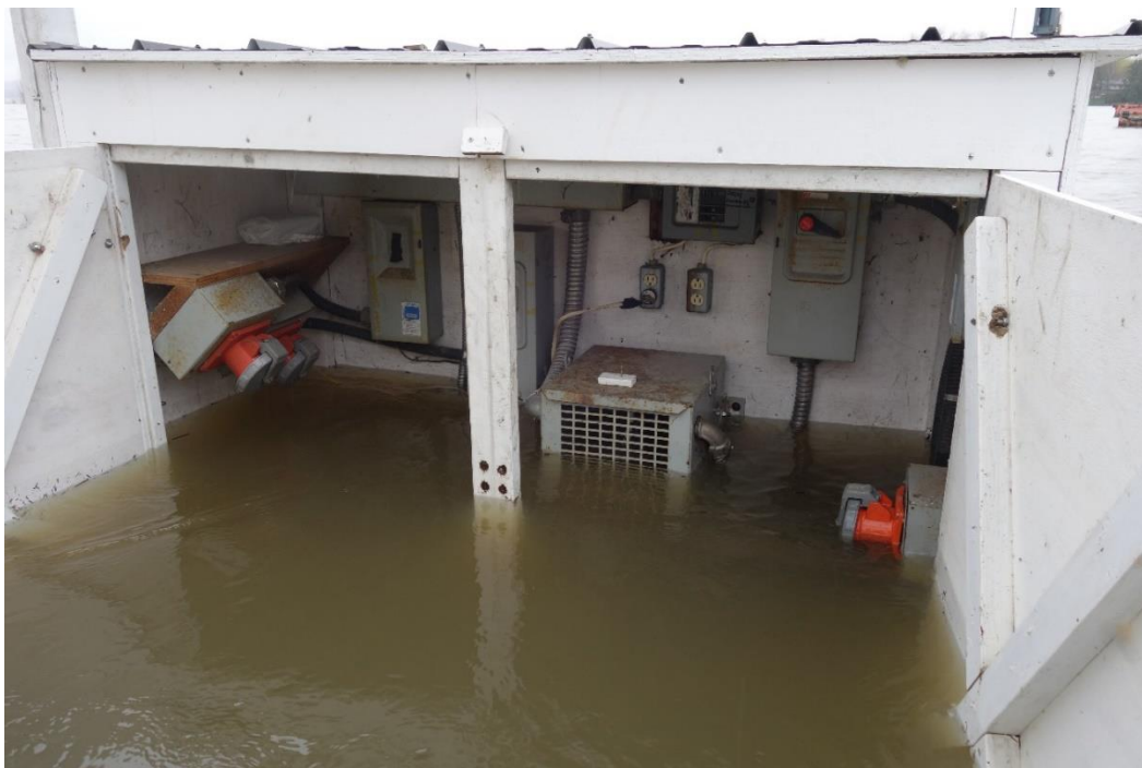
Image 6: Submerged electrical system. (Photo Credit: Anonymous, Club de Voile Deux-Montagnes)
