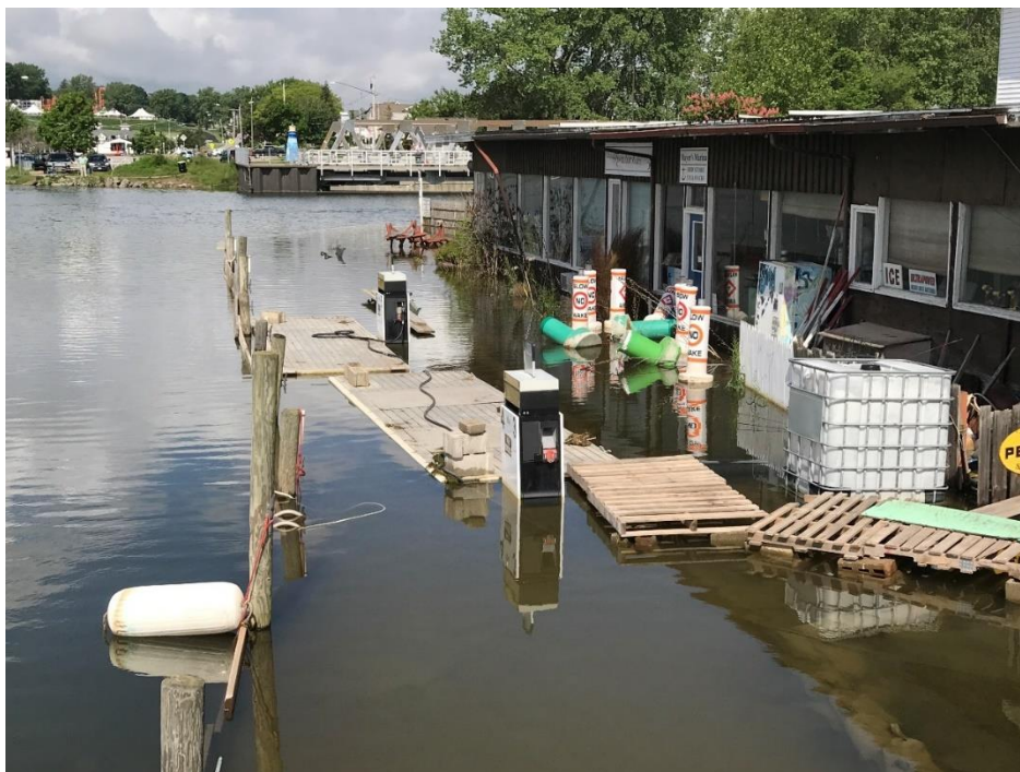
Image 10: Marina seawall underwater. The waves from boats kept hitting building. (Photo Credit: Allison C. Mayer, Mayer's Marina Inc.)
