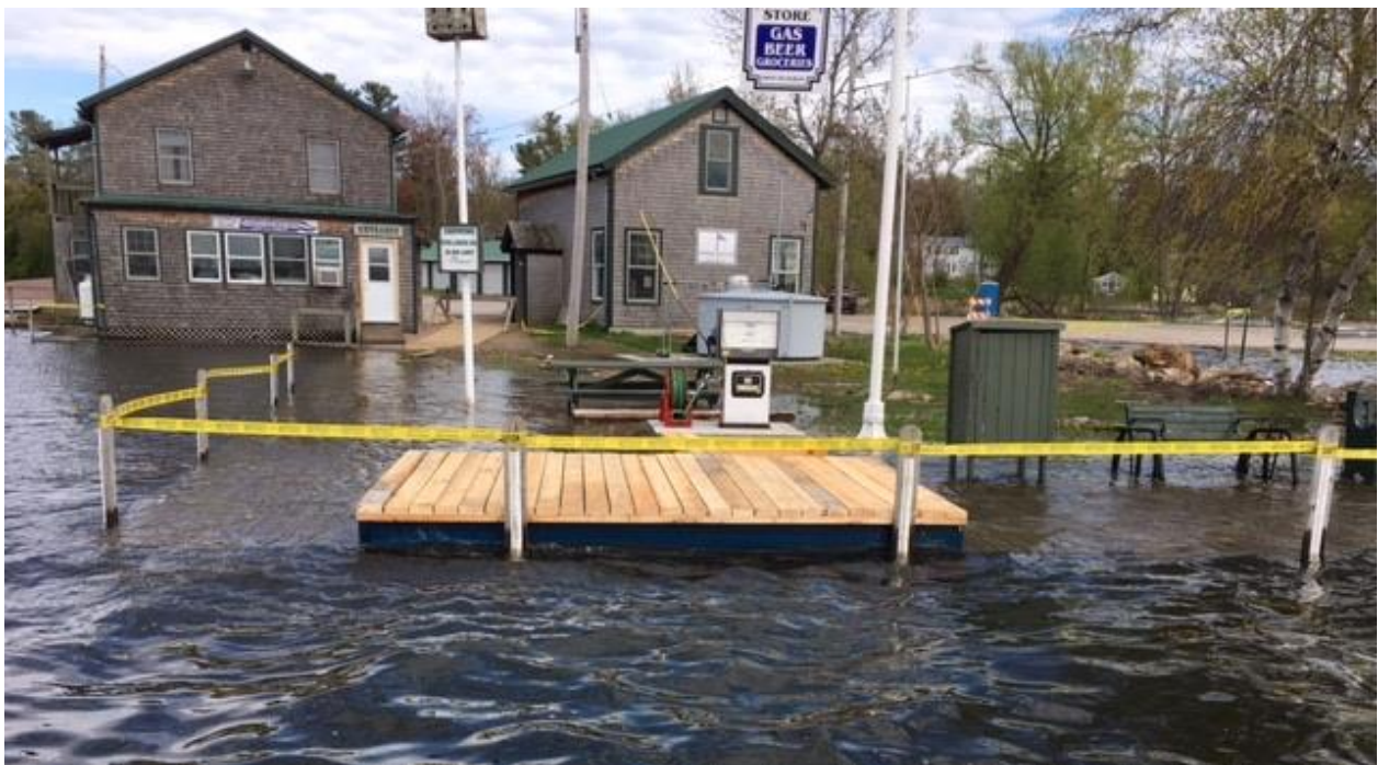
Image 11: Damage to public gas dock (Photo Credit: Anonymous, Chippewa Yacht Club)
